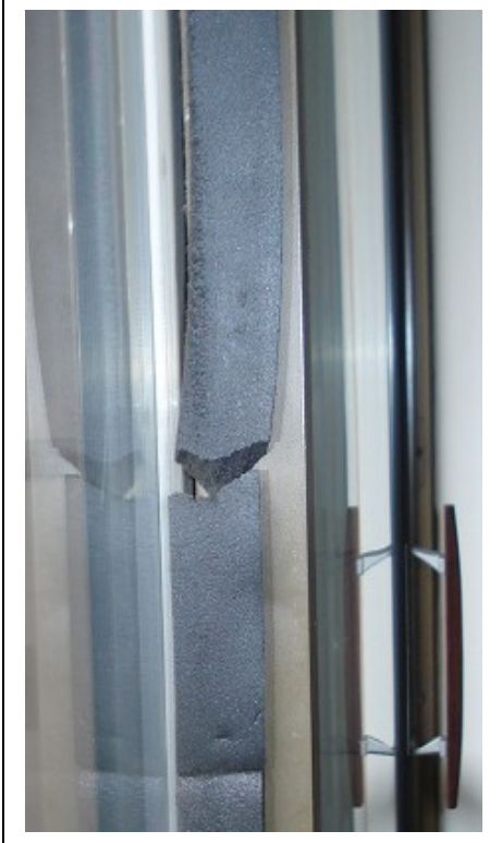
Attempts to seal the sliding glass doors have been ineffective
