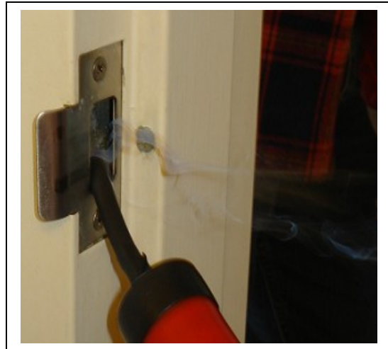
The door jambs are so leaky that many residents have inserted makeshift plugs to reduce the draft.
