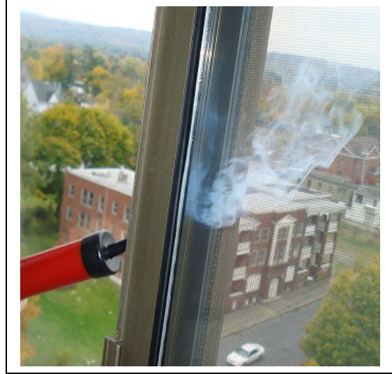
The windows need weather-stripping...
