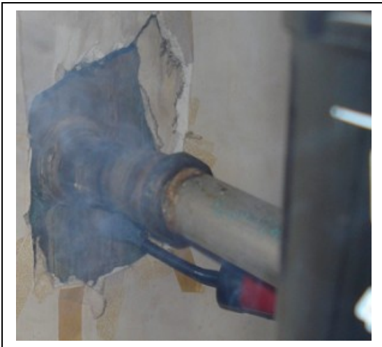
Lower mechanical room pipe chases need sealing.
