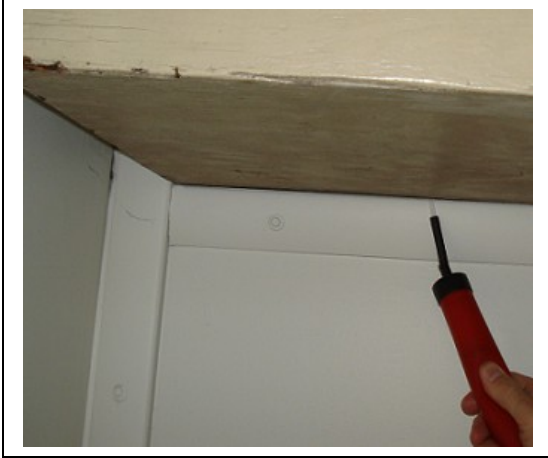
Leakage paths in common areas include the perimeter of this air-conditioner cover.
