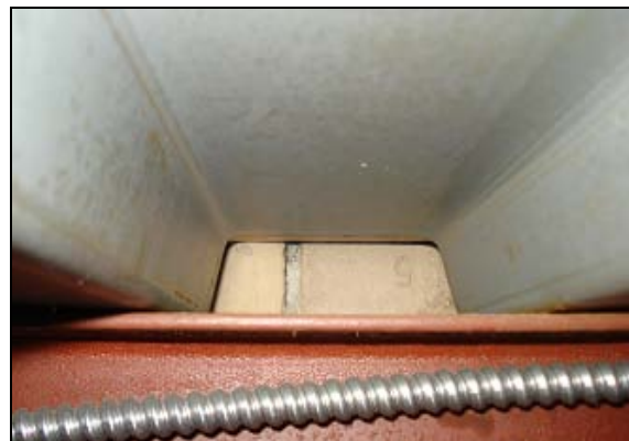
The roof/wall joint in the original building has a quarter-inch gap.
