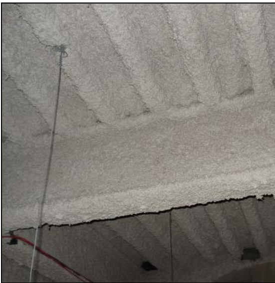
The roof deck in the addition has been insulated, sealing most of the roof/wall joint.
