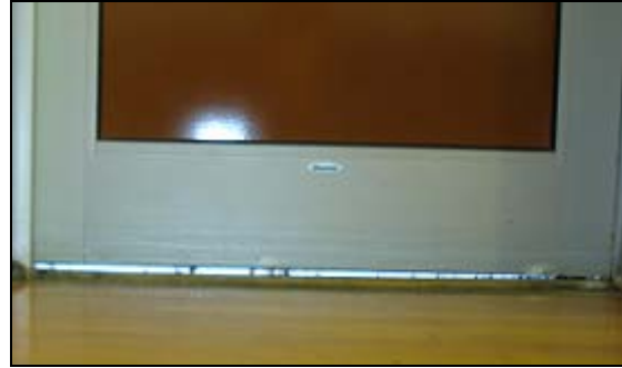
Daylight can be seen where a door sweep has failed.
