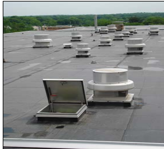
Rooftop ventilators need perimeter sealing.
