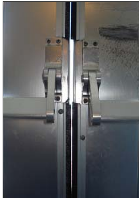
Here, the weather-stripping is new, but it does not have the correct profile for the door.
