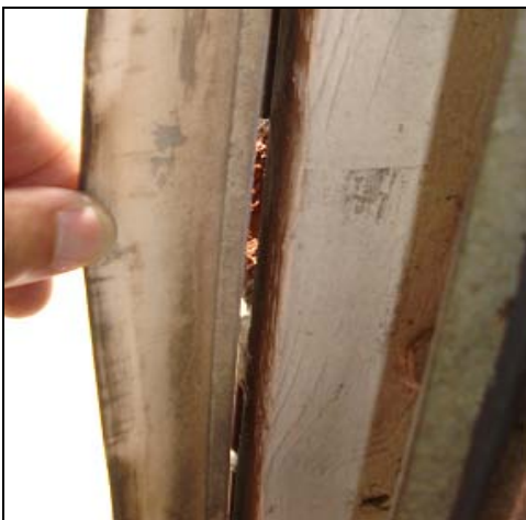
Ineffective weather-stripping on a overhead service door's perimeter.
