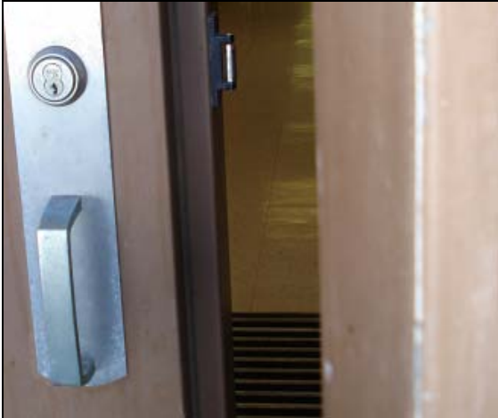
Most of the doors lack weather-stripping.
